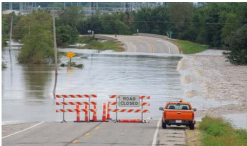
Floodwaters cover rural roadway blocked by a work truck and "Road Closed" barricades. (source TTI)
